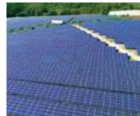
S-05 Hokota Solar Power Plant
