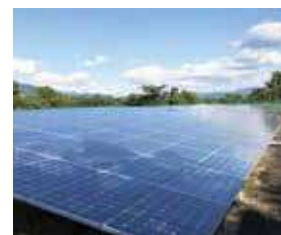
S-08 Shinshiro Solar Power Plant
