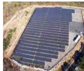
S-04 JEN Kusu Solar Power Plant
