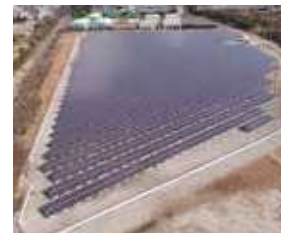
S-03 JEN Hofu Solar Power Plant
