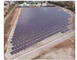
S-03 JEN Hofu Solar Power Plant
