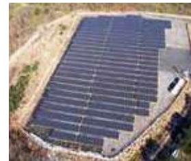
S-04 JEN Kusu Solar Power Plant
