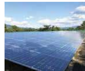
S-08 Shinshiro Solar Power Plant
